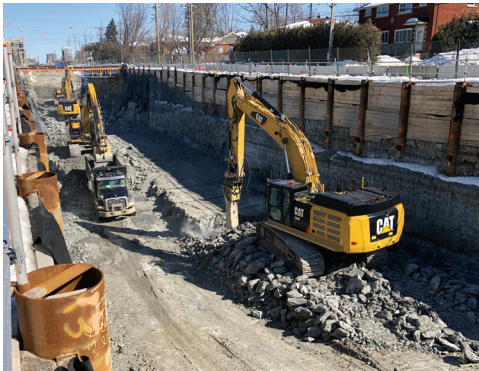
Crews have reached the full station depth of 10 meters at the future New Orchard Station.
